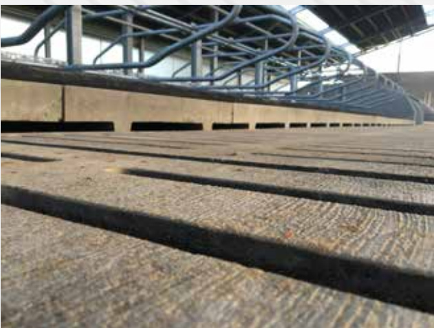
Cubicle beds with dung removal slots provide extra permeation for manure. Clean corridors provide a higher cow comfort.
