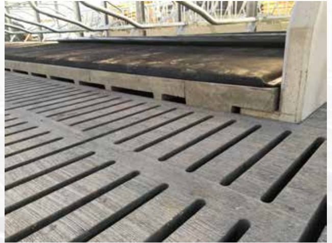
Half cubicle beds ensure that the fixations of the brackets are not on the seam of 2 plates.
